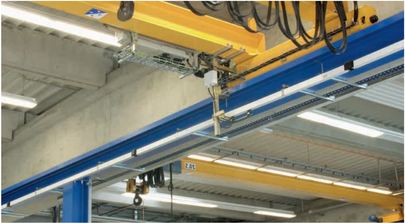
KBH Installation - Overhead Crane
