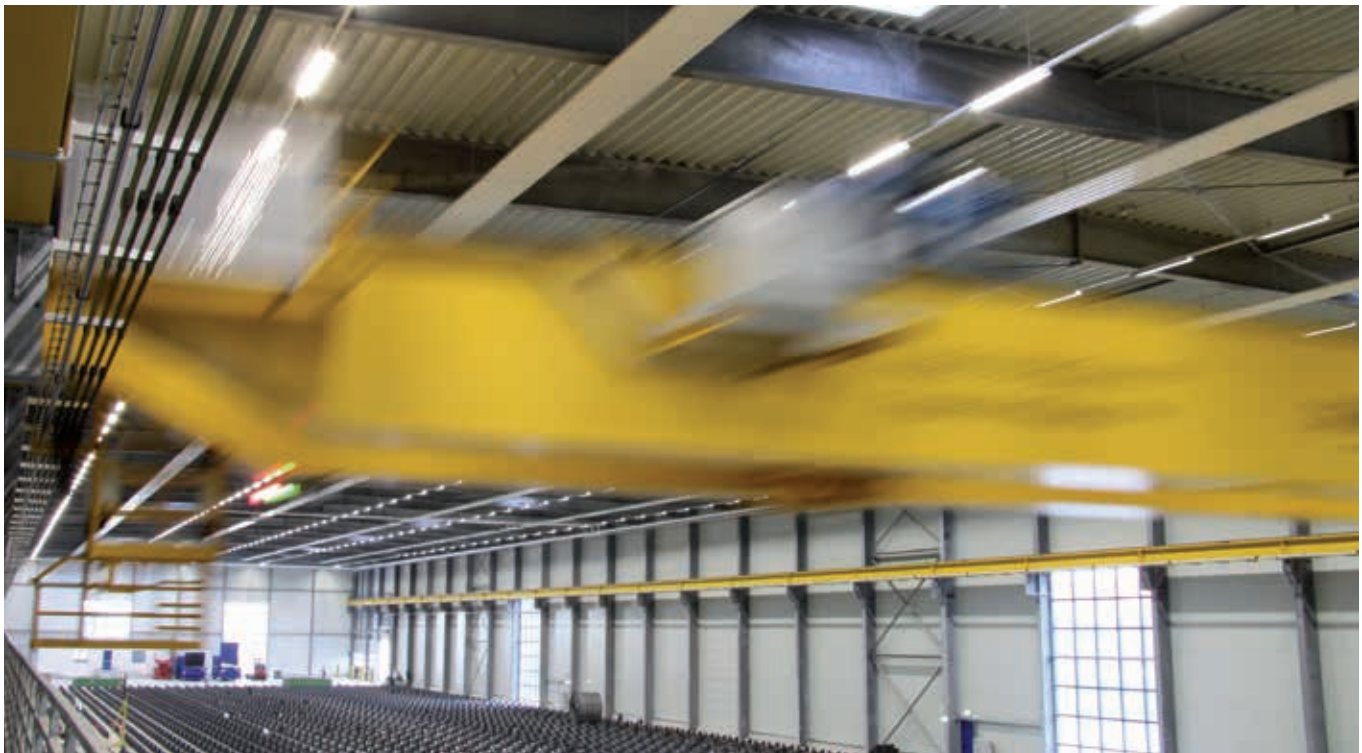
KBH Installation - Process Crane
